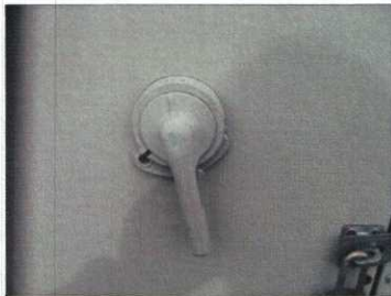
Isolating Device Location 1 Disconnect on unit
